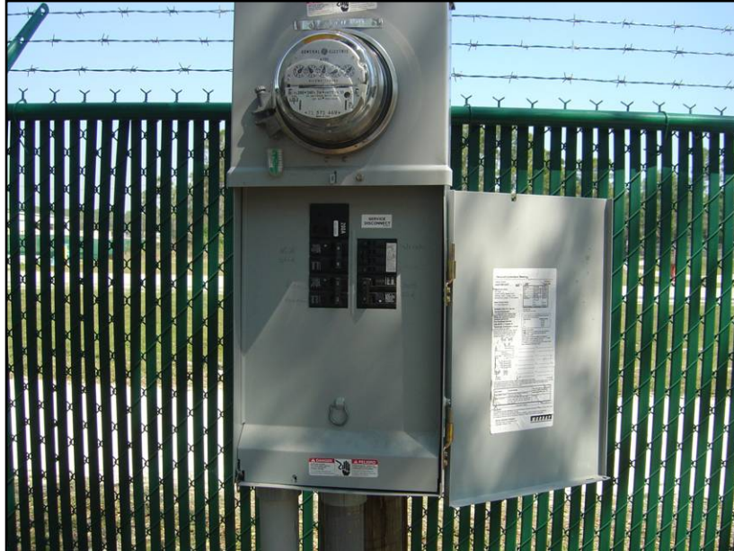
Figure 15 – Maintenance Building Power Shut-off
