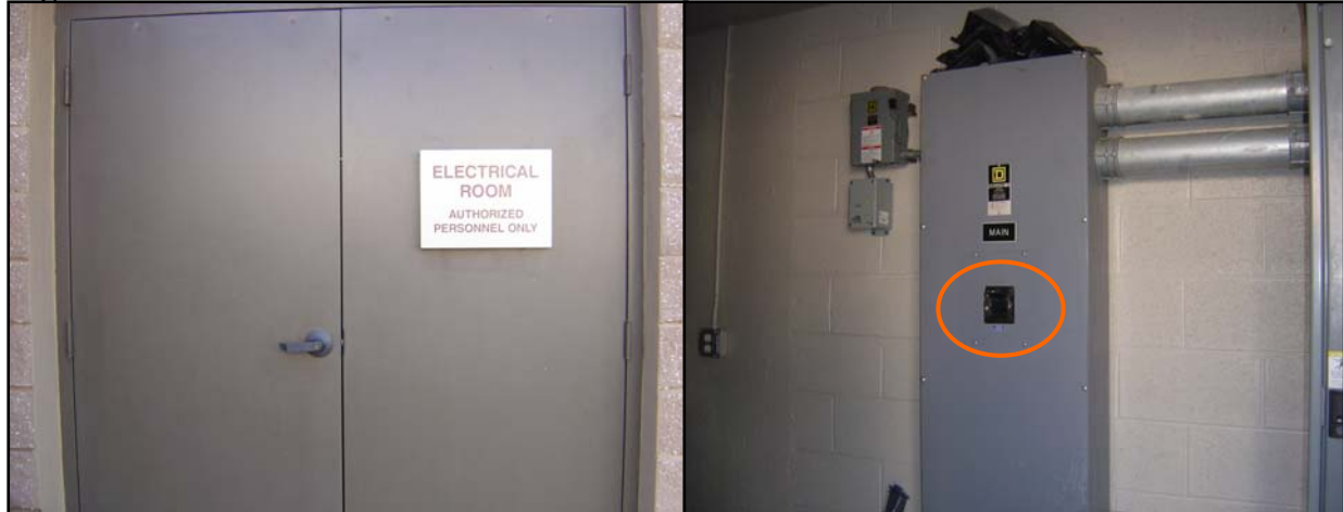
Figure 13 – Curatorial Power Shut-off
