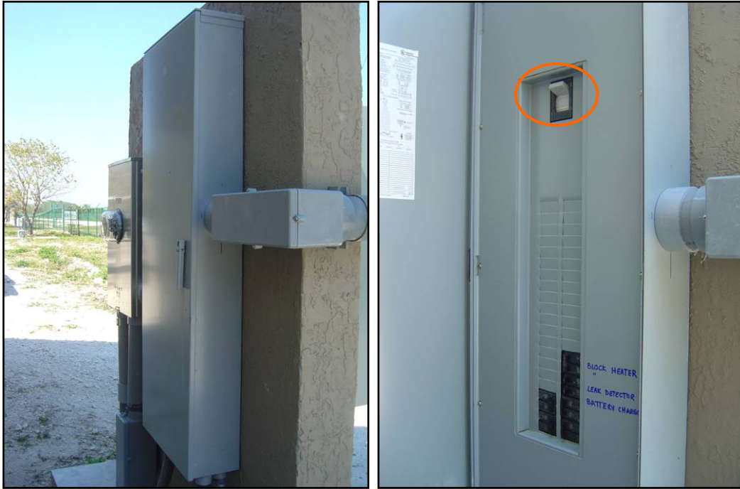
Figure 14 – Administrative Trailer Power Shut-off
