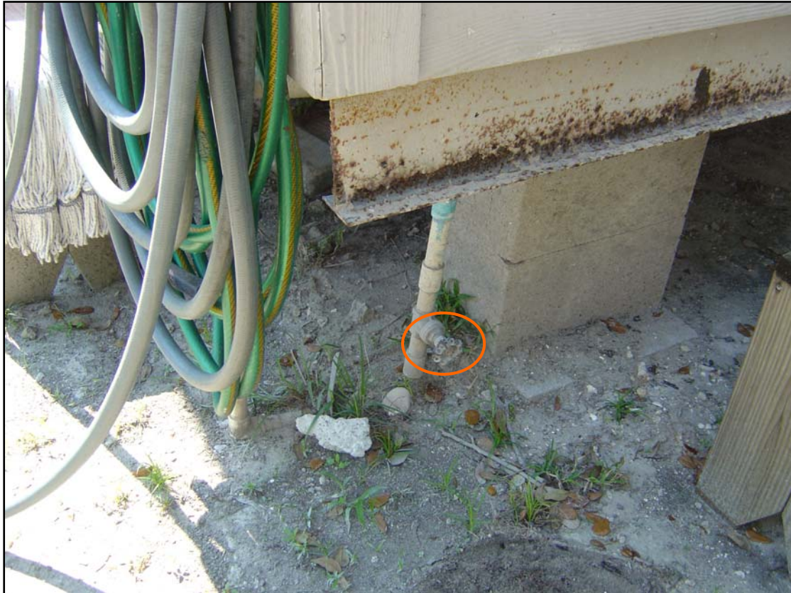
Figure 11 – Maintenance Building and Restroom Trailer Water Shut-off Valve
