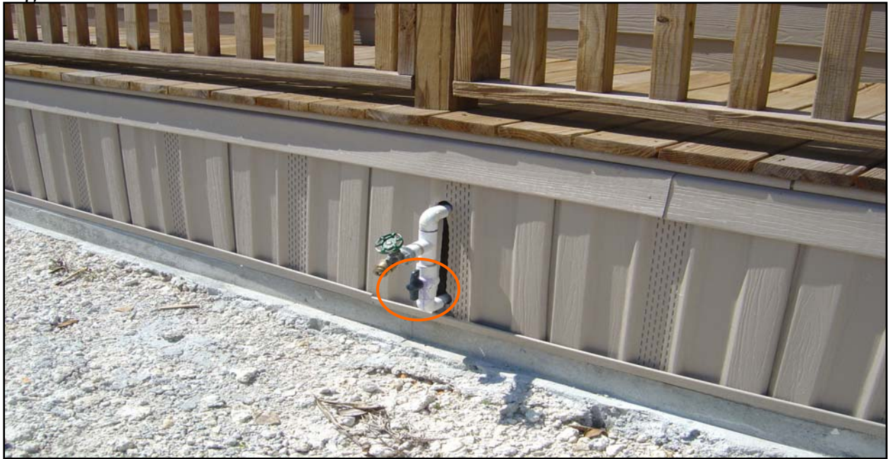
Figure 10 – Administrative Trailer Water Shut-off Valves
